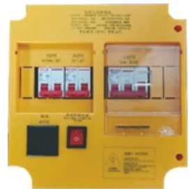
AIEC-DYX-01 Machine room power supply box
